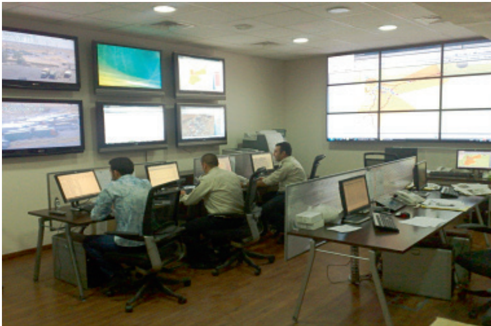
Figure 3: Main Control Room
